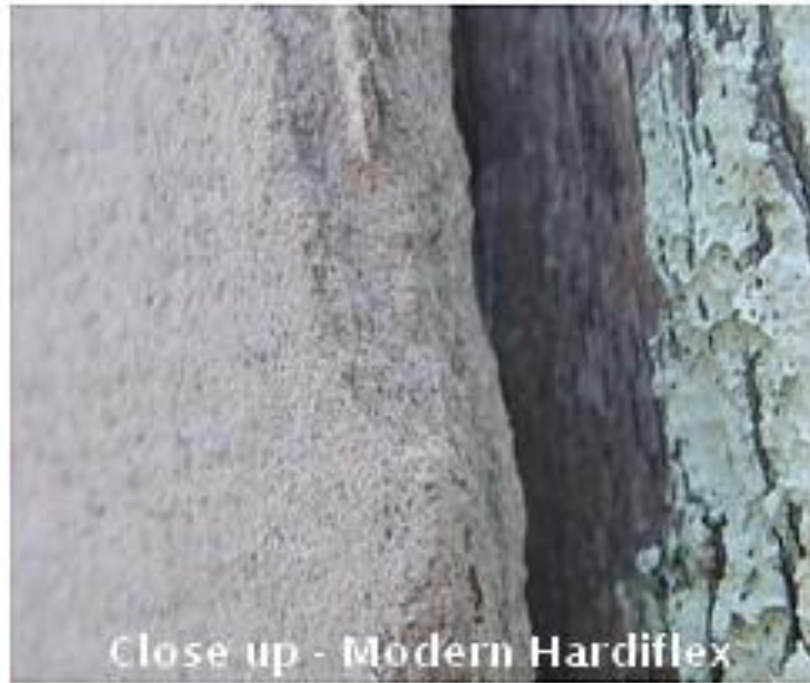
Close up - Asbestos Fibro
